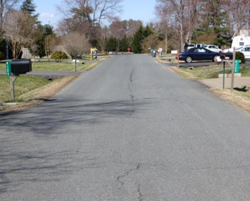
Fatigue Cracking - Low
