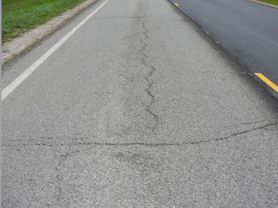
Longitudinal & Transverse Cracking - Low
