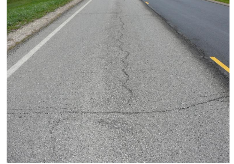
Longitudinal & Transverse Cracking Low
