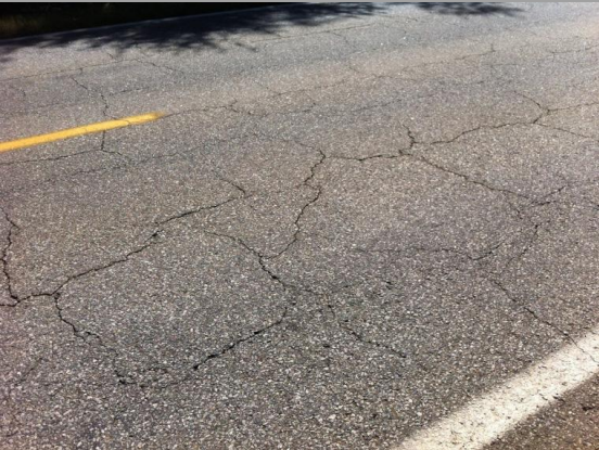
Longitudinal & Transverse Cracking
