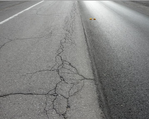
Fatigue, Longitudinal & Transverse Cracking
