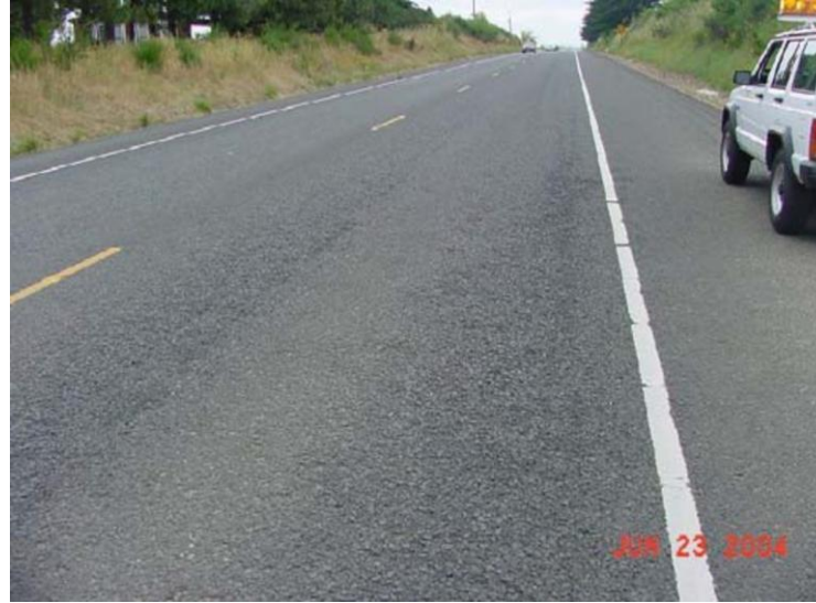
Oxidation and Raveling Moderate
