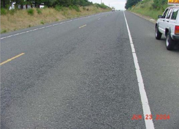
Oxidation and Raveling – Moderate
