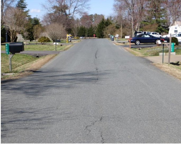
Fatigue Cracking Low
