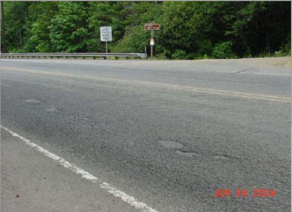
Oxidation and Raveling – High
